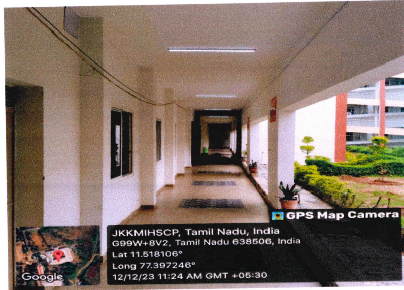
PHOTO OF LED BULBS IN MAIN BUILDING
