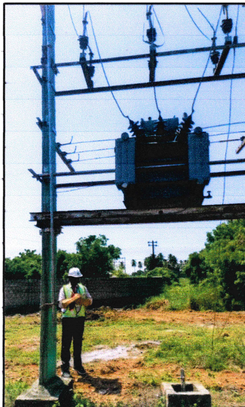
Transformer Facility in the Campus
