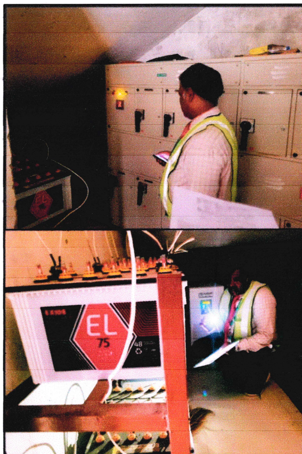
Power rooms and UPS Facility in the Campus
